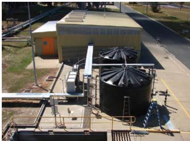
Hypochlorite dosing plant and truck unloading bay
